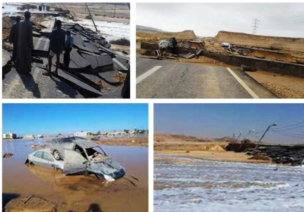
Figure 1. Photographs show destruction of El Geish Highway by March 2020 flash flood. Source: https://www.youm7.com (Online Newspaper published in 14 March 2020).
