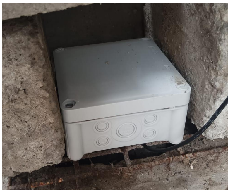
Figure 6. A sensor node located in a stormwater drain for tests.
