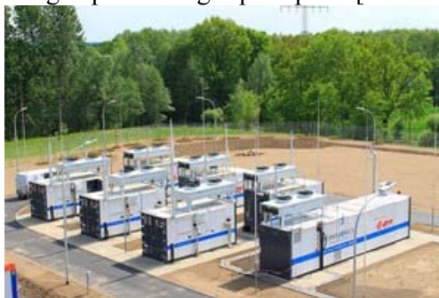
Figure 1: Falkenhagen power-to-gas pilot plant [GlobeNewswire 2013].
