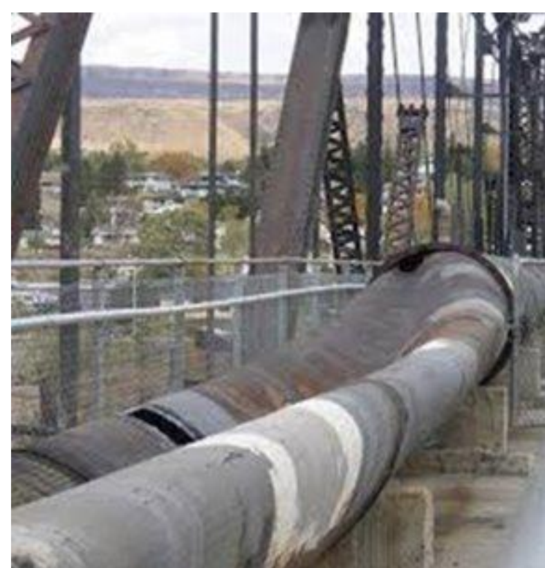
Failure due to vacuum pressure
