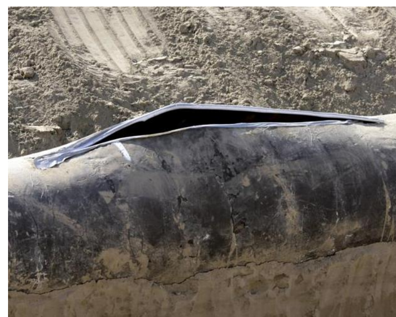
Failure due to overpressure
