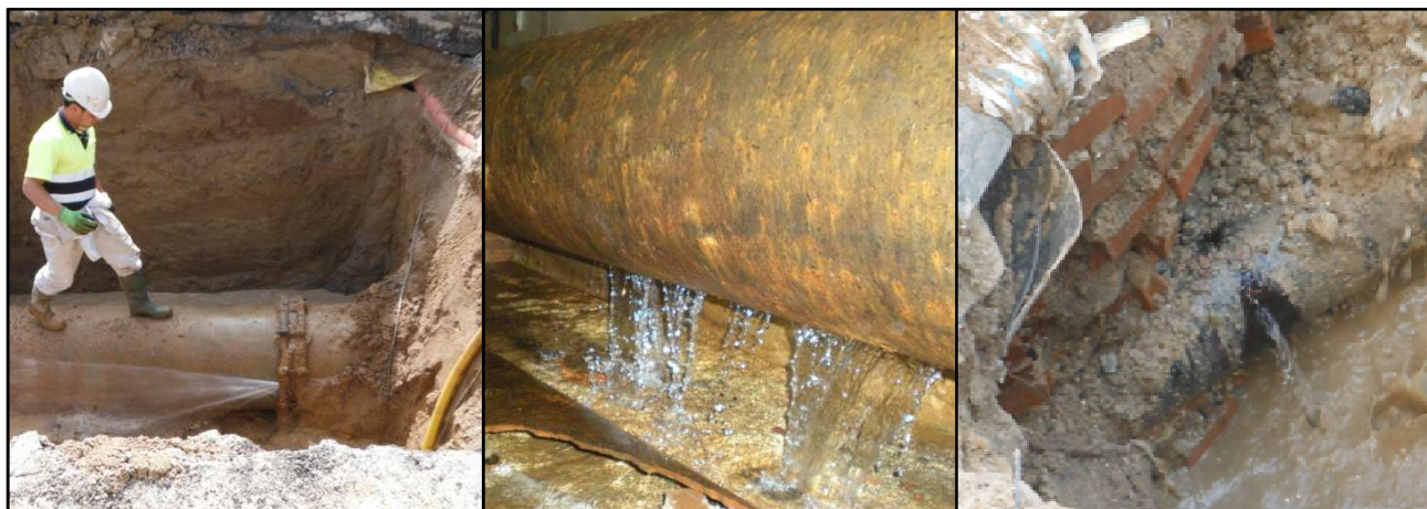
130 Figure 1. Field visits to water network failures.
