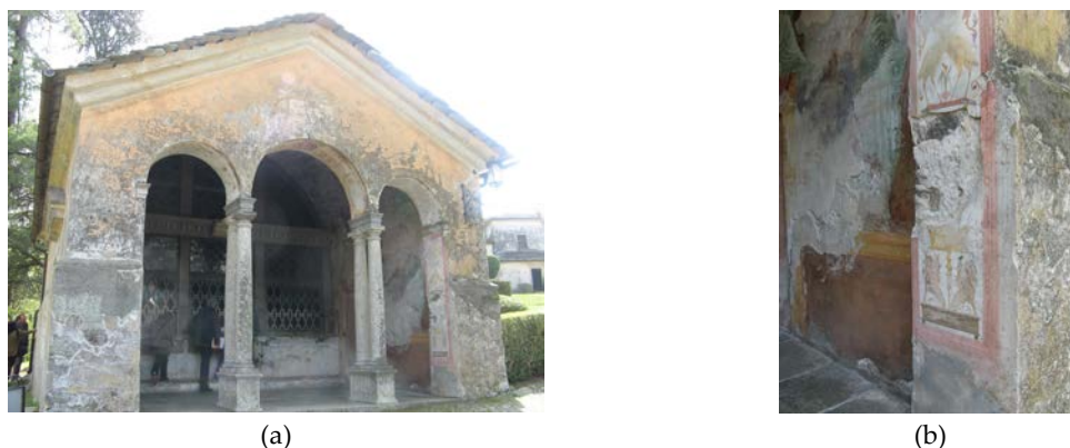
Figure 1. Chapel of the Temptations (a), and delamination problems of the historical plasters (b)
