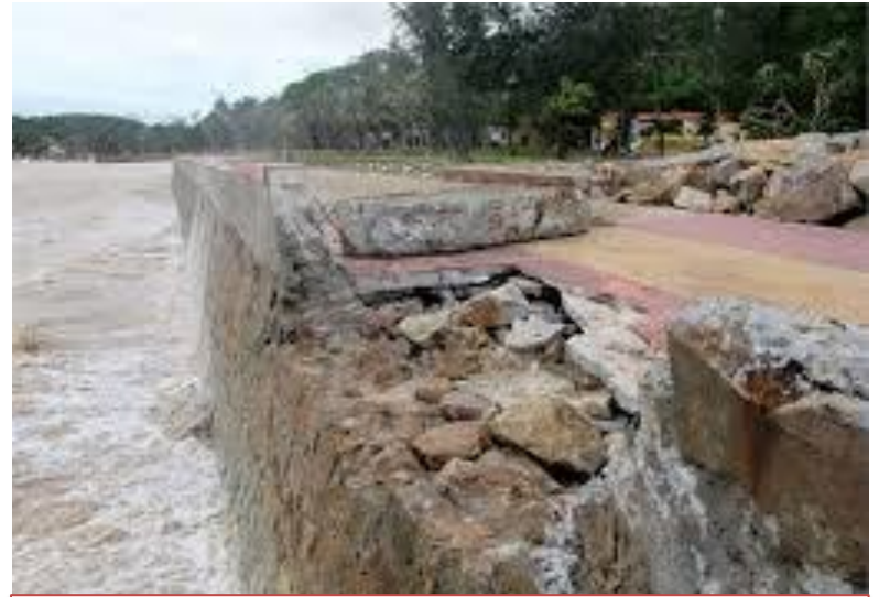
Damage after storm
