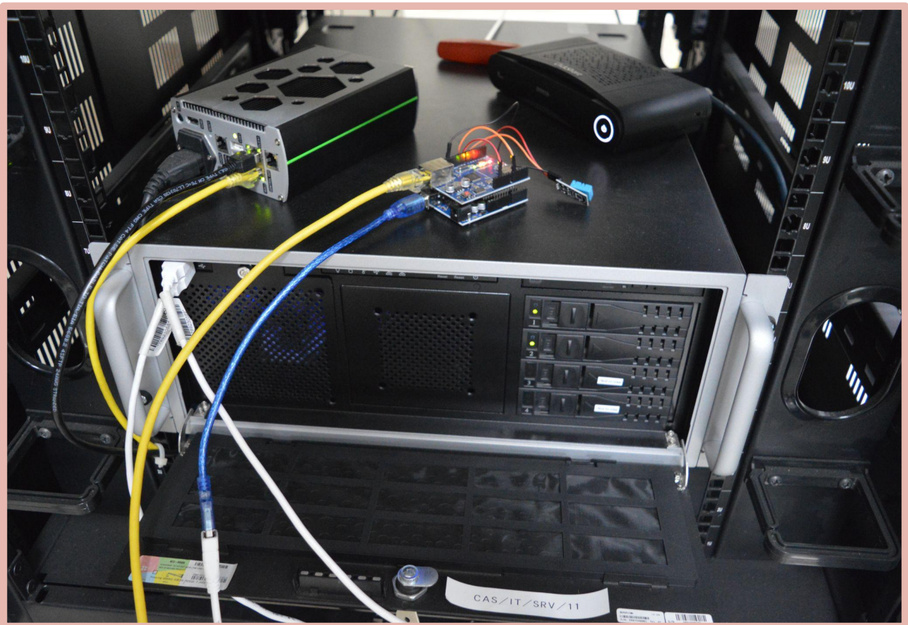
Figure (viii) - The Arduino board and DHT11 setup in the server rack of the Data center.
