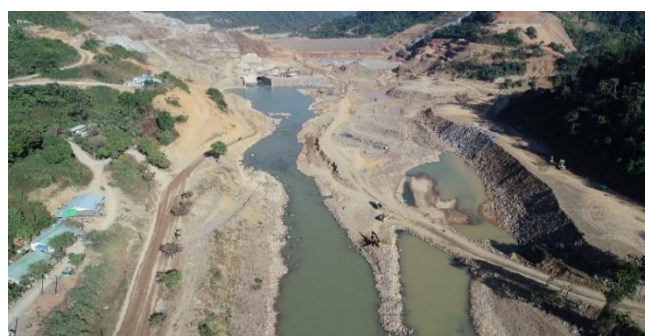
Figure 2. Construction site of the Tha Htay Hydropower project from downstream view. (Source: survey photo).
