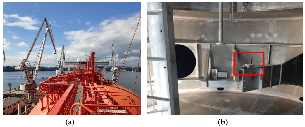
Figure 4. Gas carrier where the system was tested (a) and ORP IoT device placed inside a tank of the gas carrier (b).
