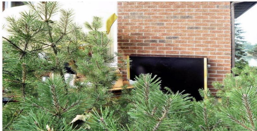
Figure 4. Air-heat exchanger. The 50 kW air-heat exchanger transfers heat into the ground loop of the test-bed system.
