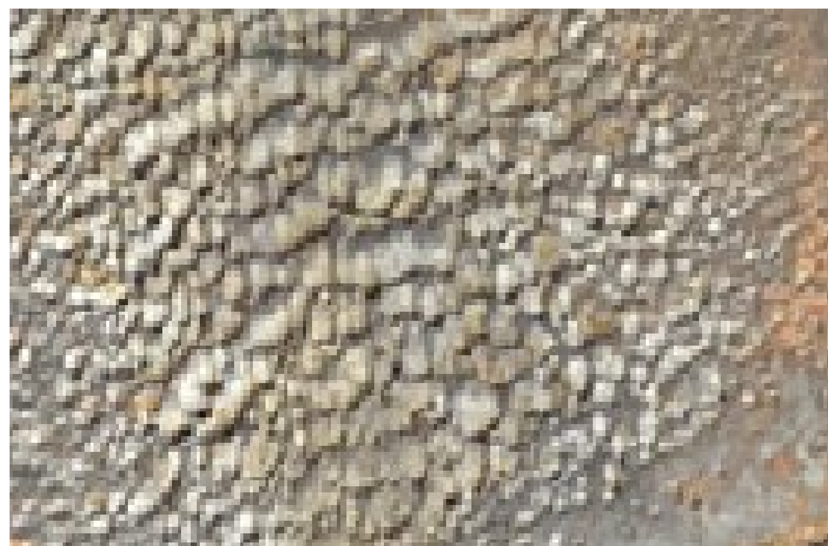
Figure 1 Observed severe pitting in 14MoV6-3 pipe
