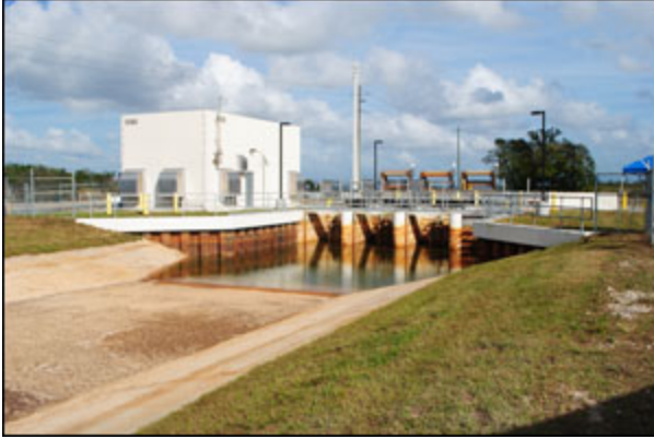
The C-111 canal pump stations became operational in early 2013.
