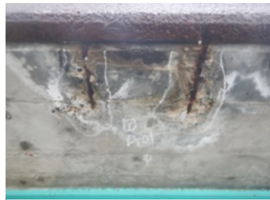
Figure 1. A typical picture of delamination (with rebar exposure)
