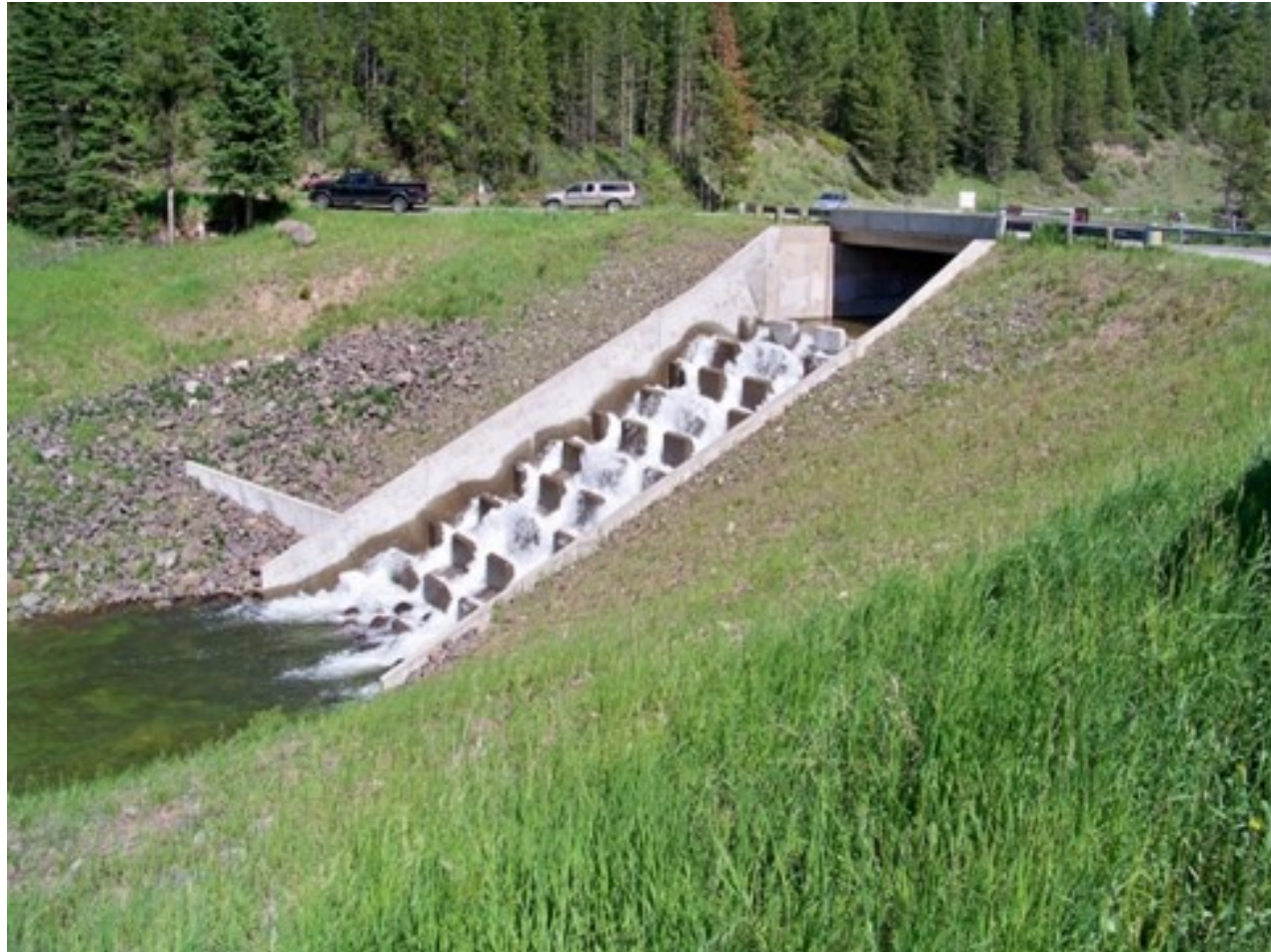
Example baffled chute spillway in Bozeman, Montana USA (photo from C. Brown).
